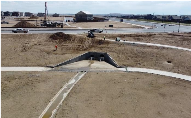
Pond C Forebay 3 (View: West)
