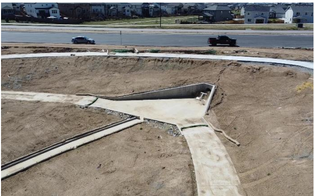
Pond C Forebay 1 (View: West)
