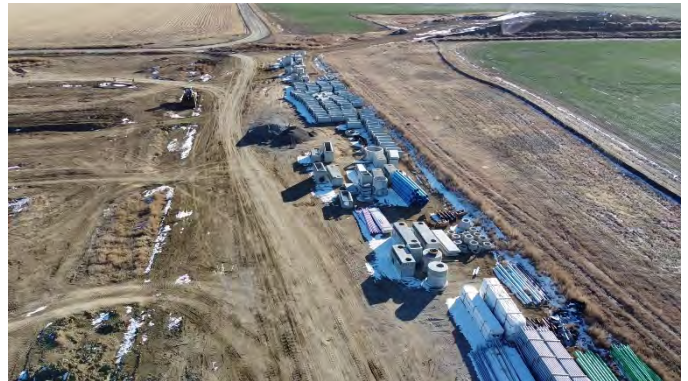
Filing 5: Stored Materials (View: East)
